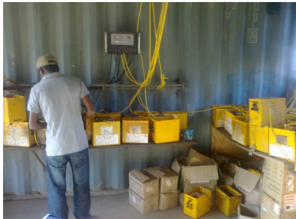
Fig. 3(b). A maintenance center of SEF in Rema
